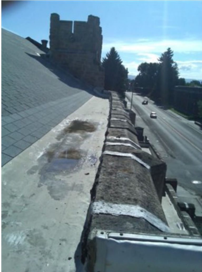
Photo 1: View of south clerestory parapet wall showing possible outward bow.
